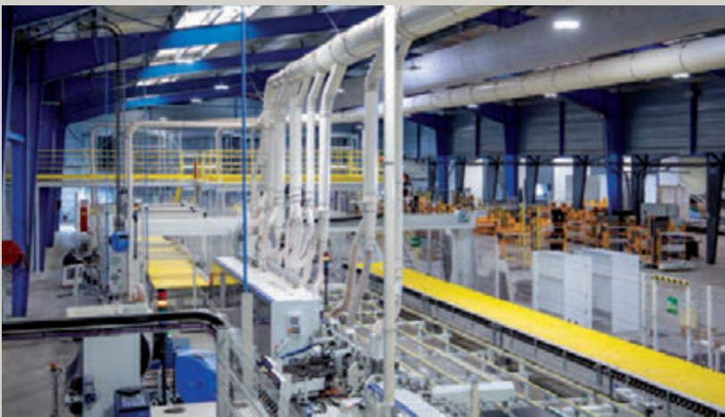
Some pictures of the Gautier plant with SCM engineering solutions.
